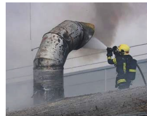
Flue gas System
